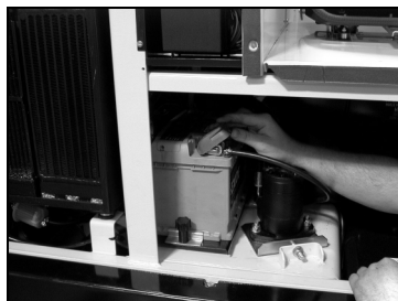
Loosen the clamp for the negative post-lead
