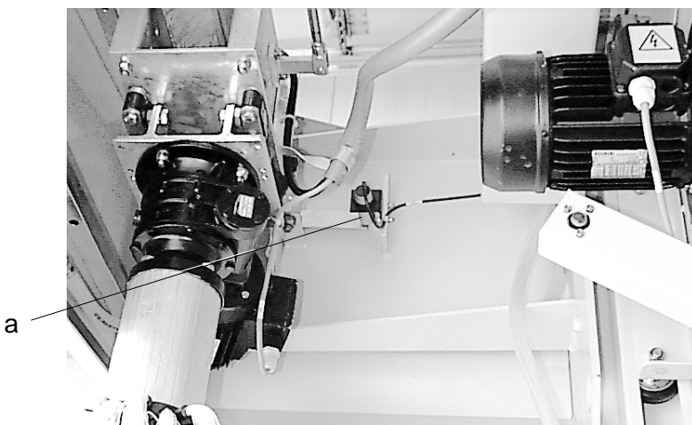
Fig F.3: Column 1 top a Limit switch swivel side brush traverse
